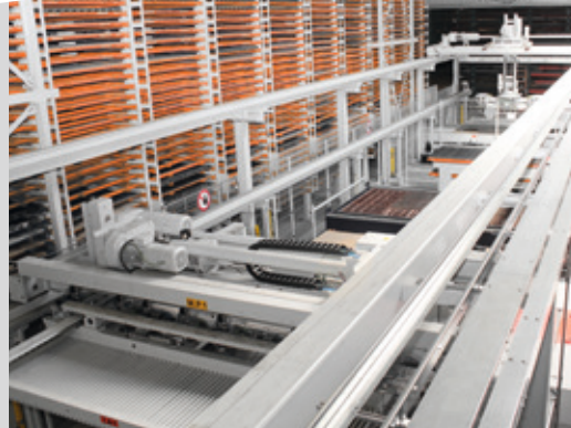
UNILINE in the sheet metal processing industry
